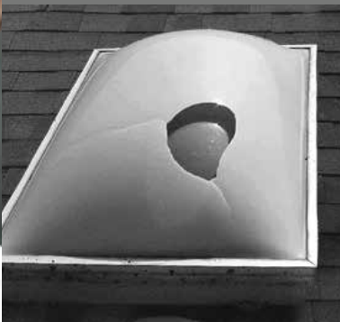
Old acrylic domes can be easily damaged.
